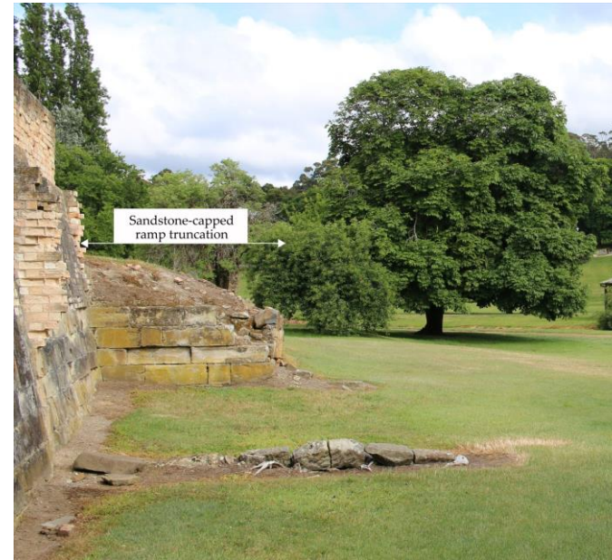
Figure 131: Looking along the Champ Street retaining wall toward the truncated end of the ramp. Note how it prominently sticks out beyond the line of the wall (facing north west)
